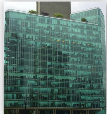
Simply meeting ASTM E 2141 results in a high probability for glare and unsightly window treatments in future years
